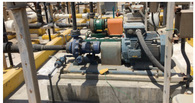
New Non-Metallic Pump as installed at Treatment-1 Hypochlorite Distribution
